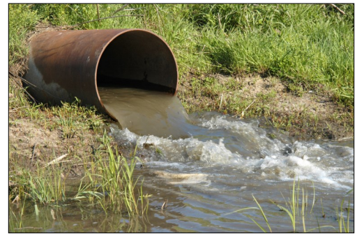
A sewage discharge pipe (not at Cuddington)
